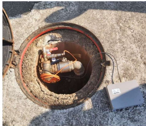
↑ ISURLOG NB on-field unit for drinkable water distribution network pressure monitoring
