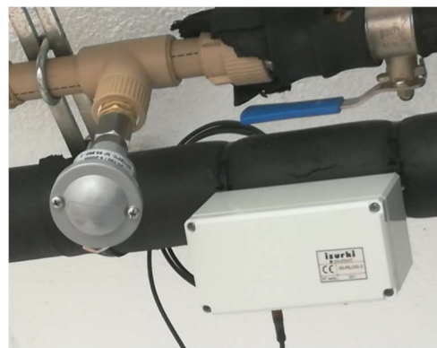
⇄ ↑ ISURLOG NB on-field unit for HVAC network temperatures monitoring at a health facility.
